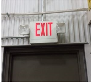
Emergency lights above door in west Bay are not working
