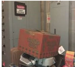
Poor housekeeping in MCC2
