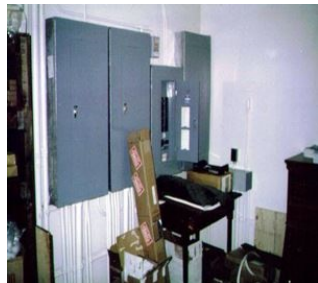
Blocked electrical panel in QA lab
