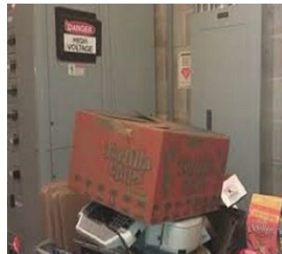
Blocked electrical panels in MCC2
