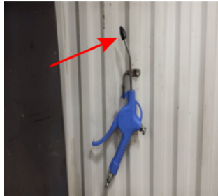
Non-compliant air nozzle
