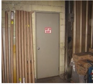
Door to storage closet in basement is properly marked NOT AN EXIT
