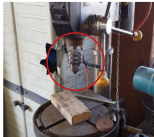
Drill press in Maintenance Shop needs a chuck guard
