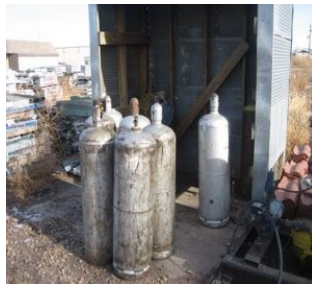
Example of cylinders NOT stored properly
