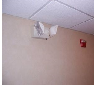
Emergency lights outside Breakroom are not working
